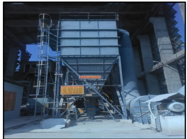
High capacity bag filters installed in the conveyor circuit
