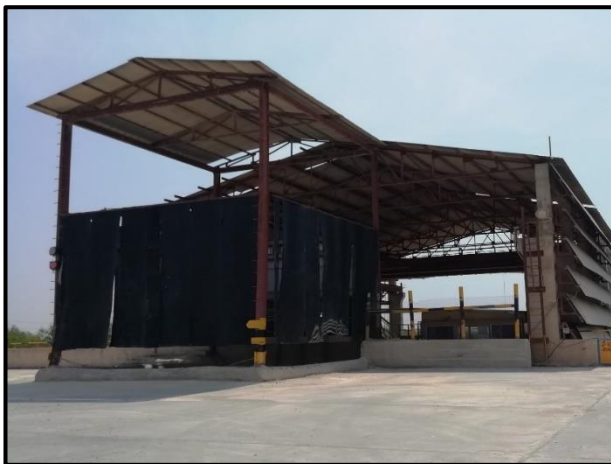
Dump Hopper Covered with belt Conveyor to arrest the dust
